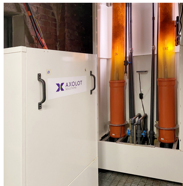
AxoPur systems in regular operations.
